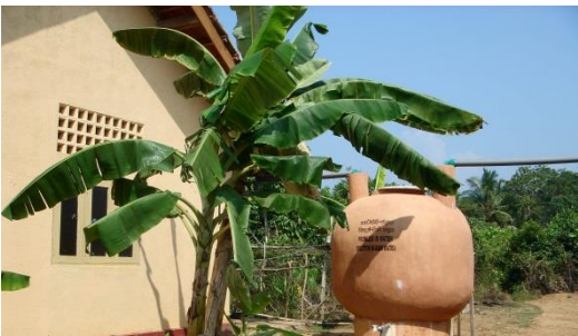
Rainwater harvesting system in Sri Lanka
