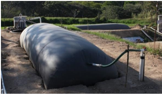
Anaerobic digester at a coffee farm in Honduras
