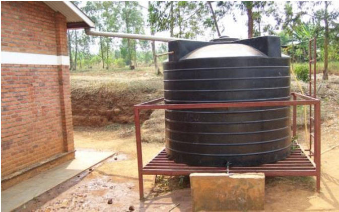
Rain-fed water tank
